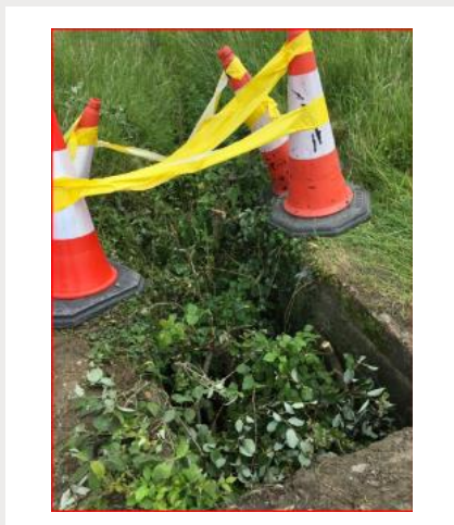
Missing void protection on highway infrastructure
