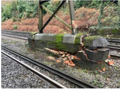
December 2023 – Damaged bridge supports
