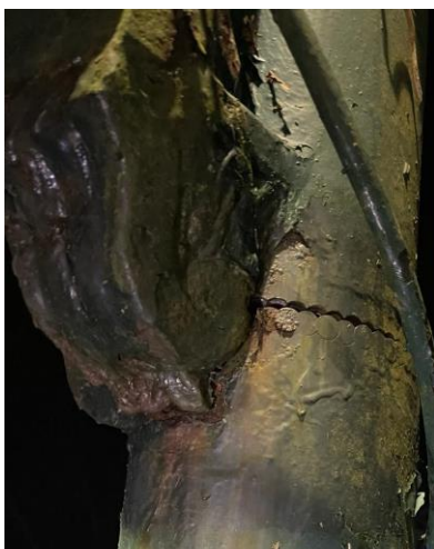
January 2023 – Fractured bridge columns
