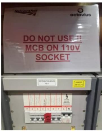
Signage installed post incident
