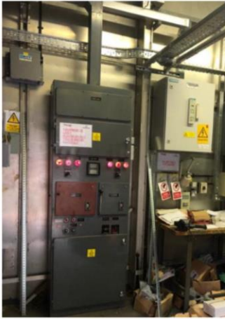
Substation Power transformer
