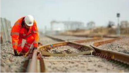
Example of damaged points ends.
