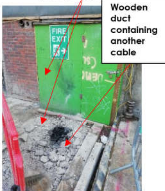
Picture 2 – Cable that was struck.
