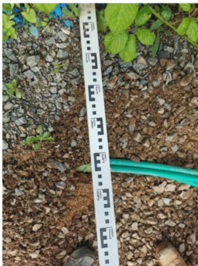
Image showing position of duct in relation to marked location as per as built information.
