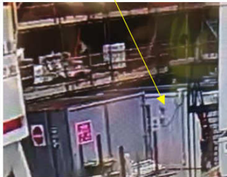
Picture 2 – Contractor office starts to be lifted as the skip (out of shot) catches it.
