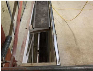
Picture 2 – Example of an unsafe covering
