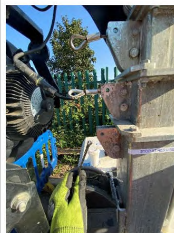
Figure 4 End of snapped cable, the other end is located within the tower mast
