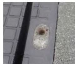
Bolt hole with stud removed
