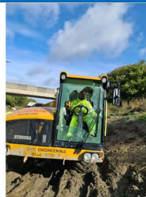
Smashed windscreen on dumper
