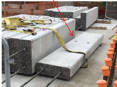
Picture 1 – Concrete Slab that fell onto the slingers foot
