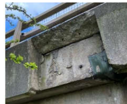
Damaged Parapet Coping
