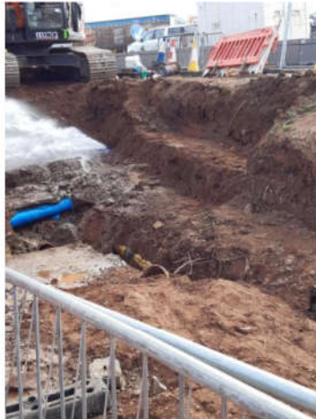
Damaged pipe releasing water
