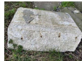
Detached Parapet Coping
