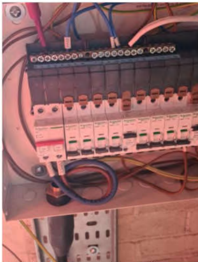
Distribution board where wiring was incorrectly installed – photo post repair
