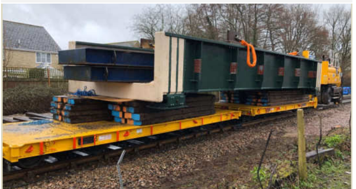
The new Network Rail standard design "U" deck ready to be lifted into position.
