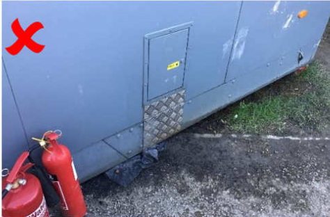
Evidence of fuel spill during the refuelling process
