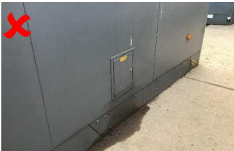
Evidence of fuel spill during the refuelling process
