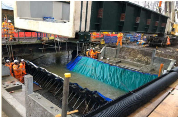
Bearings attached to the U-deck ready to be lined up with pockets in the cill beams.
