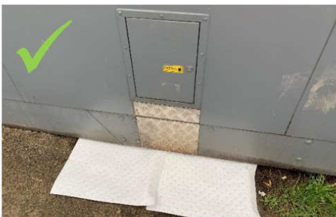
Spill nappy placed below/against the unit whilst refuelling
