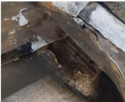
Fire damage to Polycarbonate
