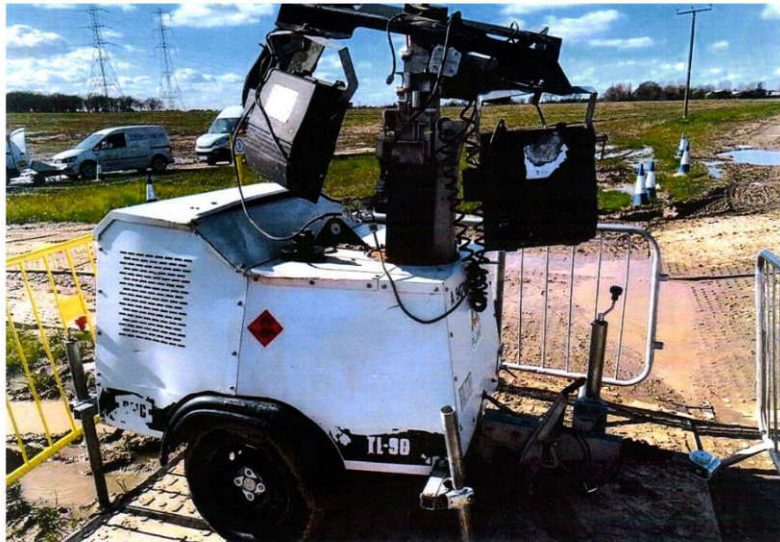
Lighting tower after the incident
