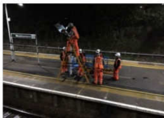
Working at height is a common rule breach. No one in the group challenged the use of a stepladder which had been approved by a construction director.
