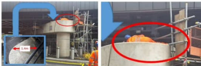
Working at height 1.4m from the edge with no protection – is it worth it?
