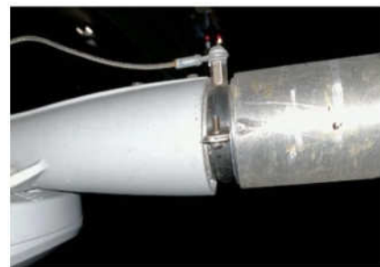
Photograph 1. Lanyard incorrectly fitted
