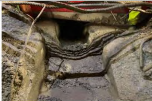
Figure 1: Damaged area with exposed rebar
