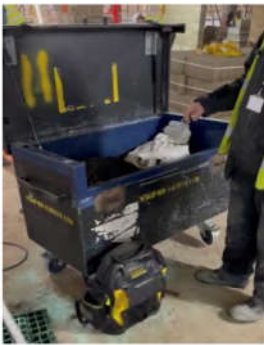
Picture 2 – Box continues to topple backwards.
