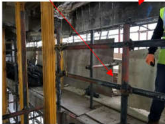
Picture 1 – Area that was being broken out. This section of the scaffold shown in the picture was not here at the time of the incident.
