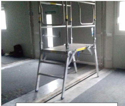
Fig. 1 – position of the single person elevated delta deck, showing exposed gap between the two modular cabins
