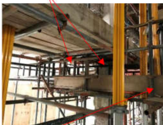
Platform that the IP fell on to.
