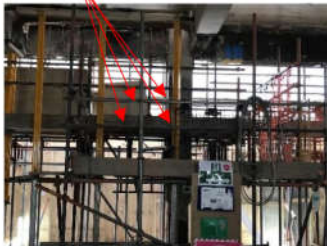
Picture 3 – scaffold beams that the loose boards had been placed on.
