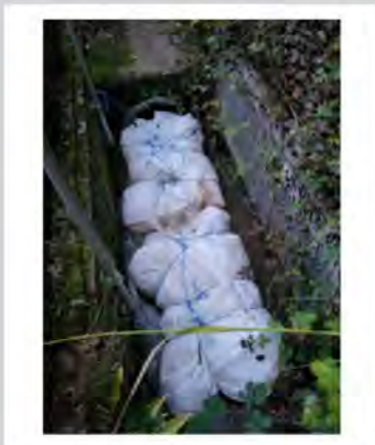
Straw bales wrapped in geotextile material as a temporary silt control measure
