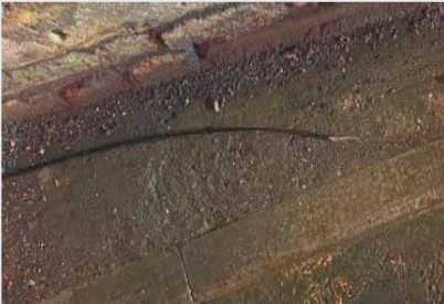
Damaged telecommunications cable
