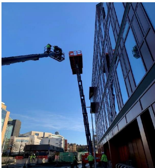
Machine angle after jack leg failure, having rotated 1.4m from the building.
