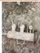
Blow out Chamber involved in the incident
