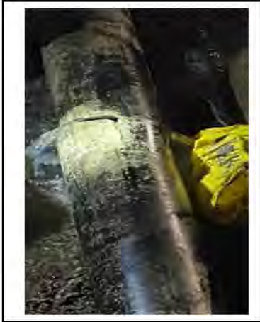
Fracture in the 9" cast iron water main
