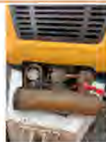
Maintained blow out chamber suitable to use
