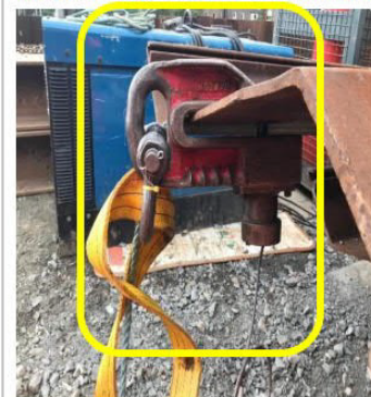
Fig. 1: Showing how the quick release Shackle was installed incorrectly (invertedly) before to the event.
