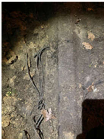
Damaged Loop cable
