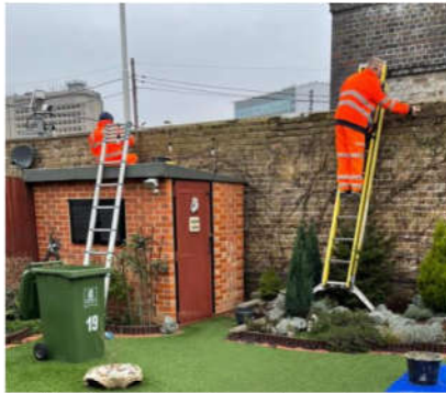
Woking – Unsafe system of work
