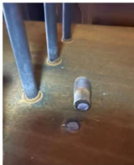
Formwork stud which appears to have failed at the weld.
