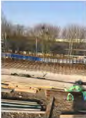
Section of scaffold type handrail removed and brickguard in place to allow anchor slab formwork installation.
