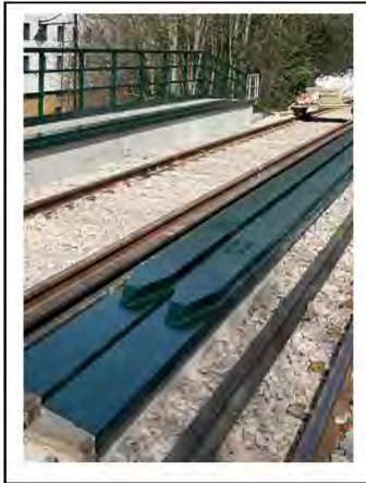
Gap in central girders
